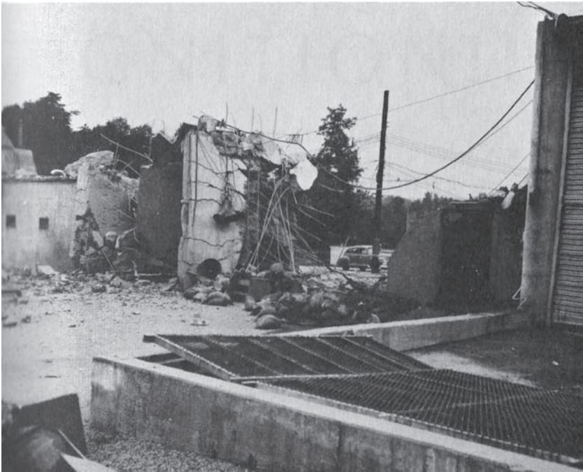
FIGURE 3 And this is what it may look like if something goes wrong. The same test cell, or its remains, is shown. U.S. Navy photo
